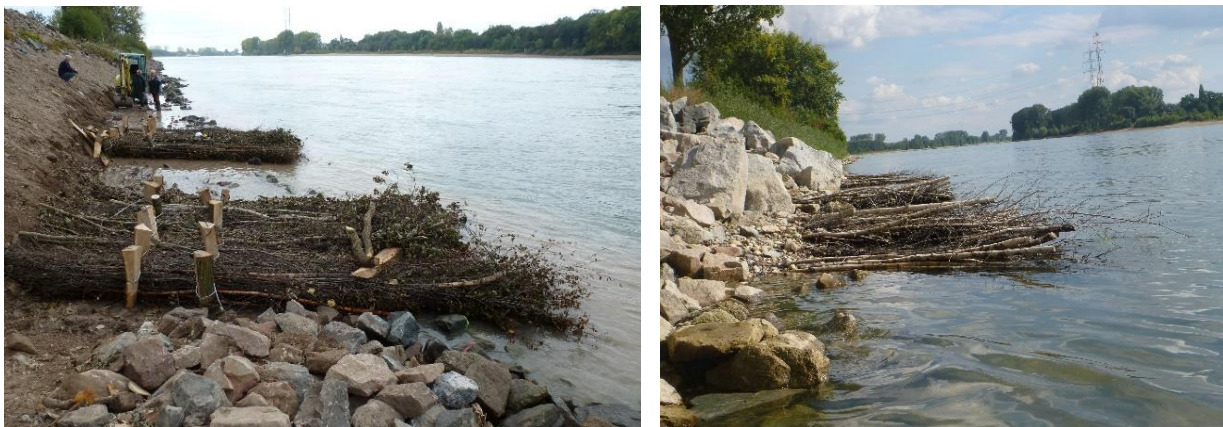
Figure 3.25: Installation of fish-effective deadwood fascines on the River Rhine, near Worms ( left , in October 2011; right , in September 2012) (Photo: K. Behrendt, BfG)
