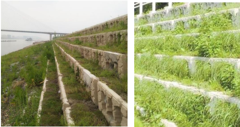
Figure 3.18: The fish-nest brick revetment (left) and with vegetation (right) along the Yangtze River
