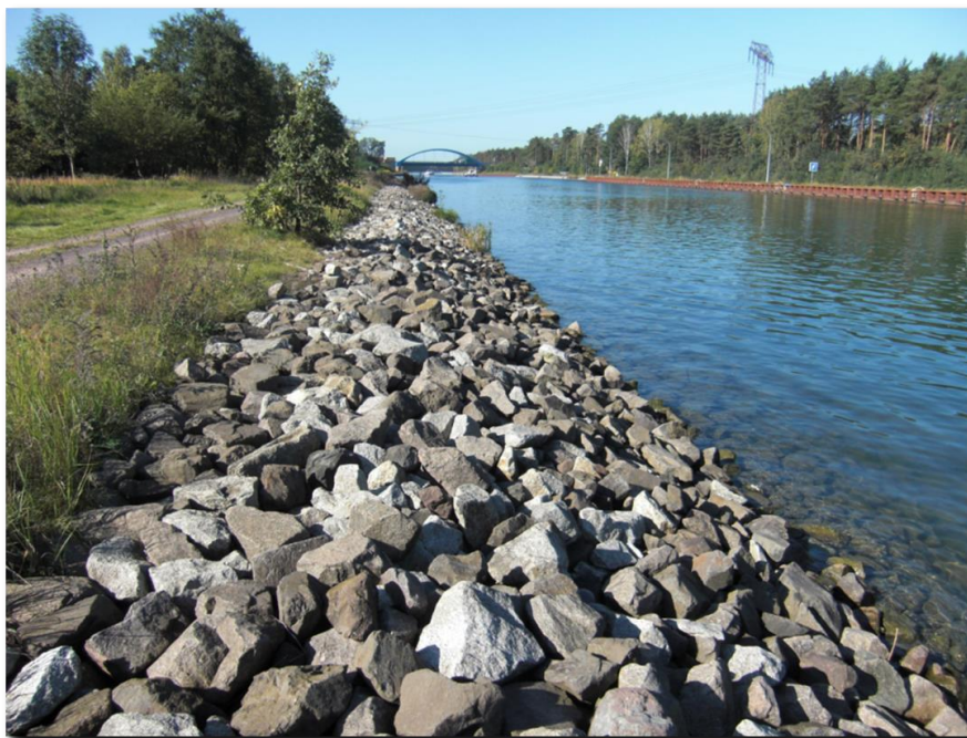
Figure 3.22: Rip rap revetment on the sloped bank in the foreground and sheet-pile wall on the opposite vertical bank (Havel-Oder-Waterway km 66)
