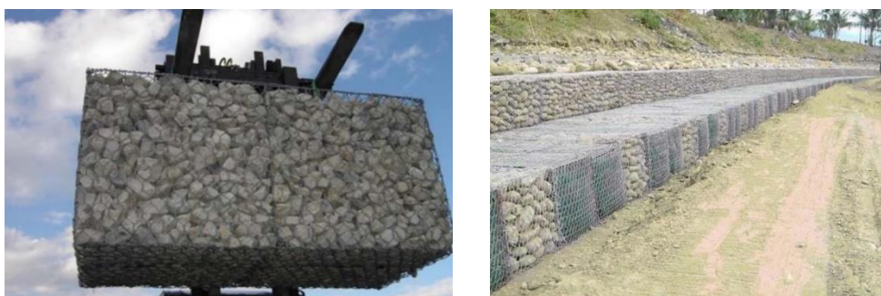
Figure 3.17: A single ecological gabion (left) and the ecological gabion retaining wall (right) in the downstream dyke section of the Three Gorges Dam
