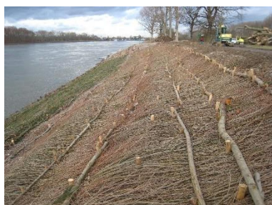
Figure 3.7: Installation of willow-brush mattresses on the River Rhine (end of November 2012) (Photo: P. Fleischer, BAW)
