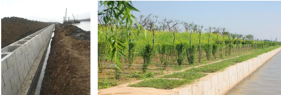
Figure 3.16: Prefabricated structures during site construction (left) and after completion (right) along the Danjin Licao River, Jiangsu, China, channel-regulation project
