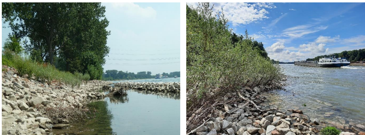
Figure 3.26: Left , creation of a stone wall in front of the bank as protection against ship-induced loading, calmed water zone with root plates behind and vegetated rip rap as TBP (River Rhine, near Worms in July 2012) (Photo: K. Behrendt, BfG); Right , establishment of a willow ridge in a rip rap bank with accumulation of driftwood (River Rhine, near Daxlanden, Germany, in August 2020) (Photo: K. Behrendt, BfG)
